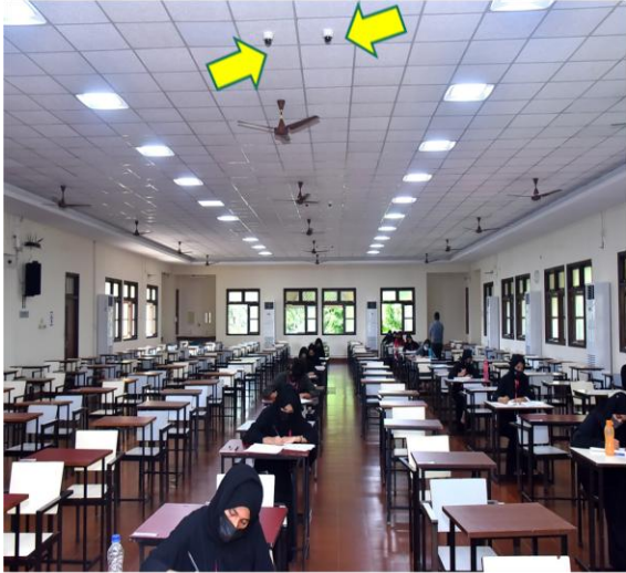
High definition CC Cameras installed in Examination halls
